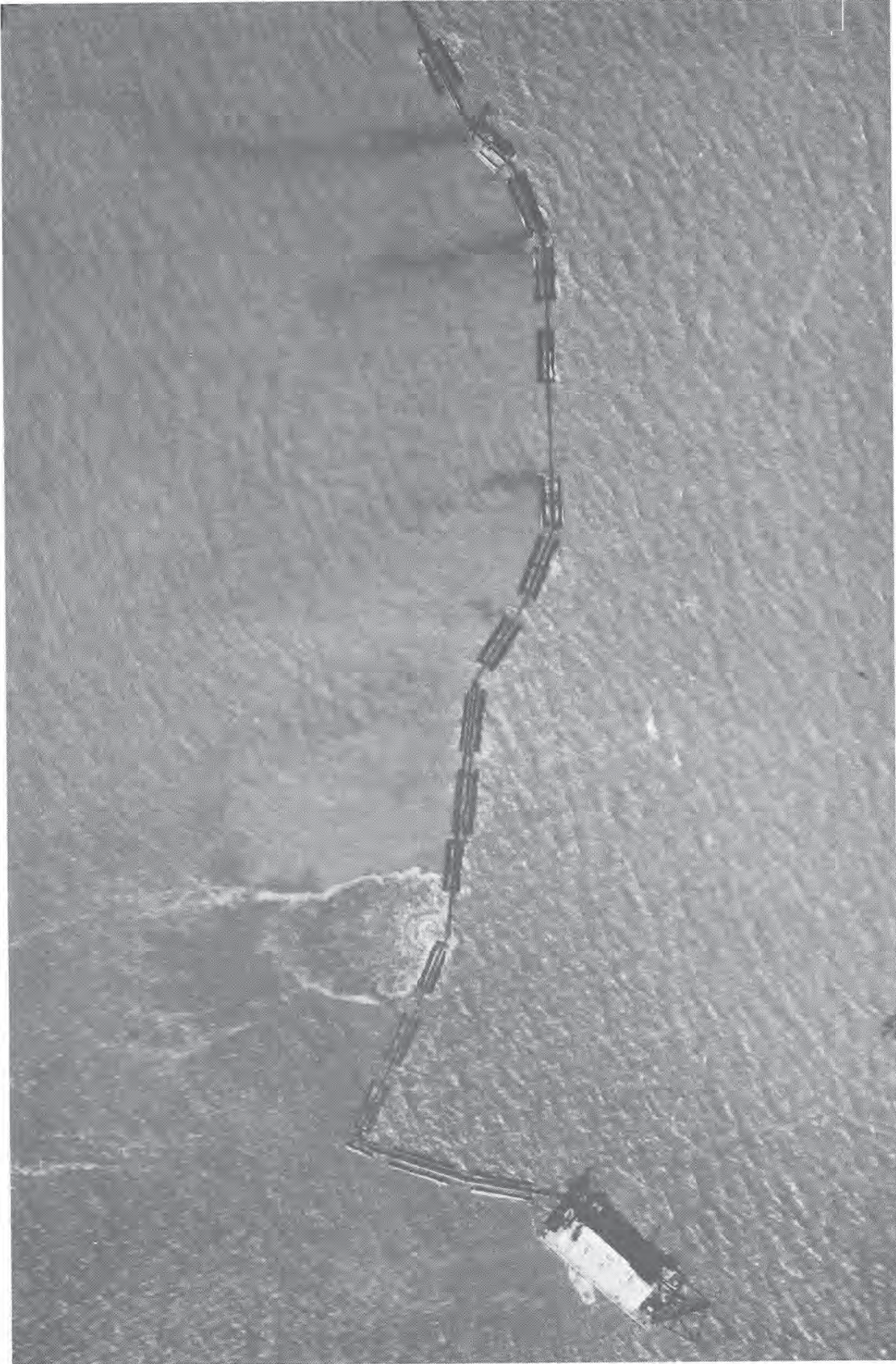
Figure 14. Turbidity creation by leaking floating line connections.
