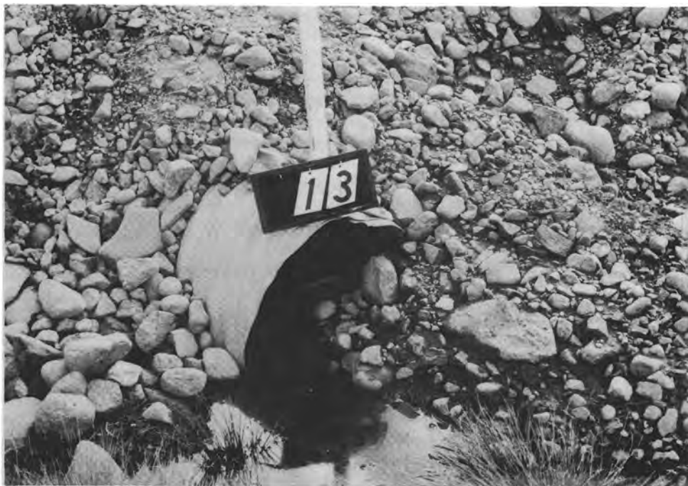
Figure 56. "Maintenance clogging" problem caused by surface material graded down sideslope of road, site 91-C2, August 1977.
