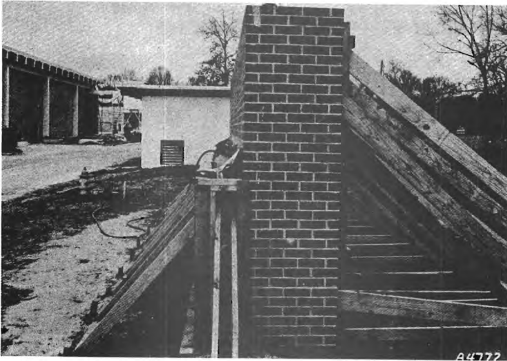
Figure 9. Wall 1. Wall deflection
