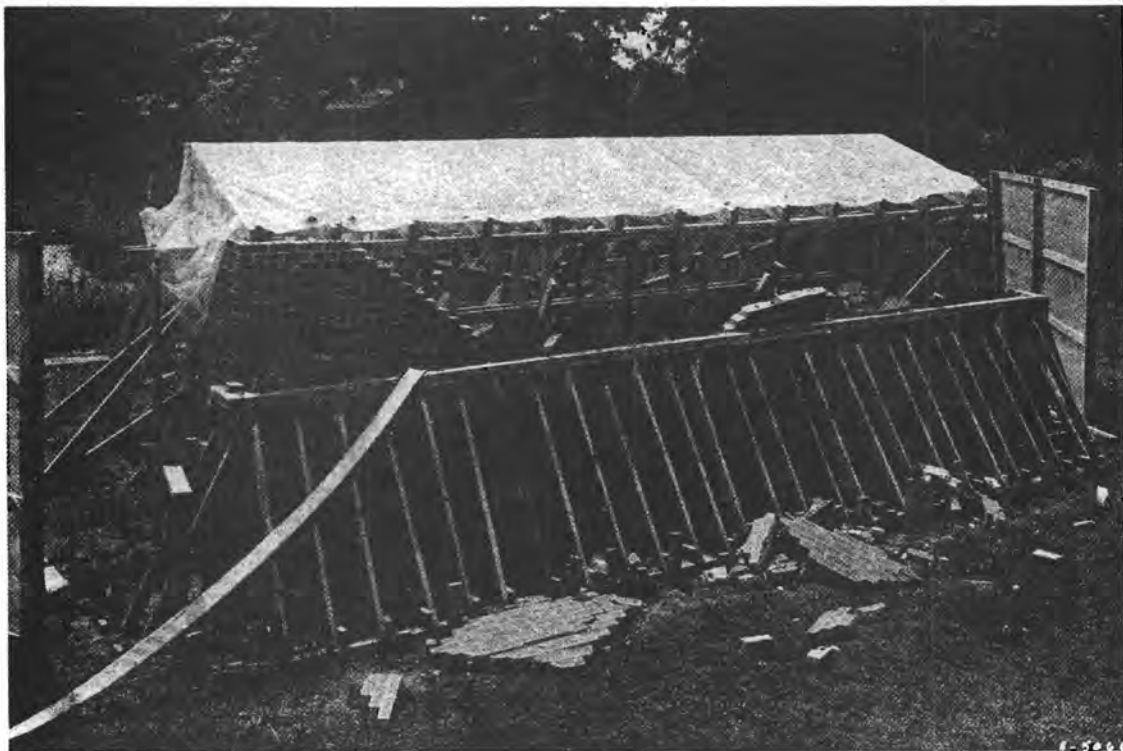
Figure 16. Wall 3. Wall failure, front view
