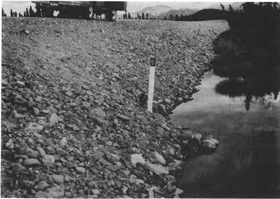
Figure 55. Upstream ponding caused by shoulder thaw consolidation and bowing of the culvert, site 91-C1, August 1977.
