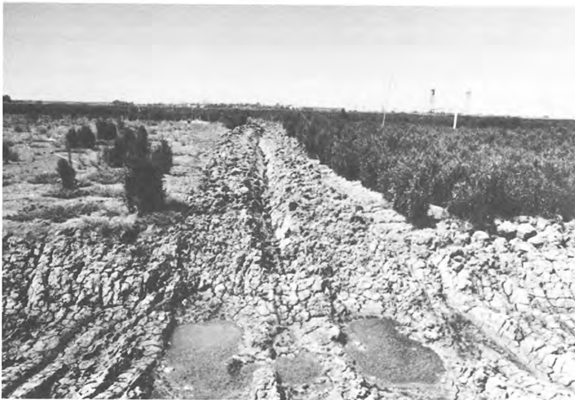
Figure 27. Thiokol drag plow produced trenches extending from the dragline perimeter trench into the disposal site
