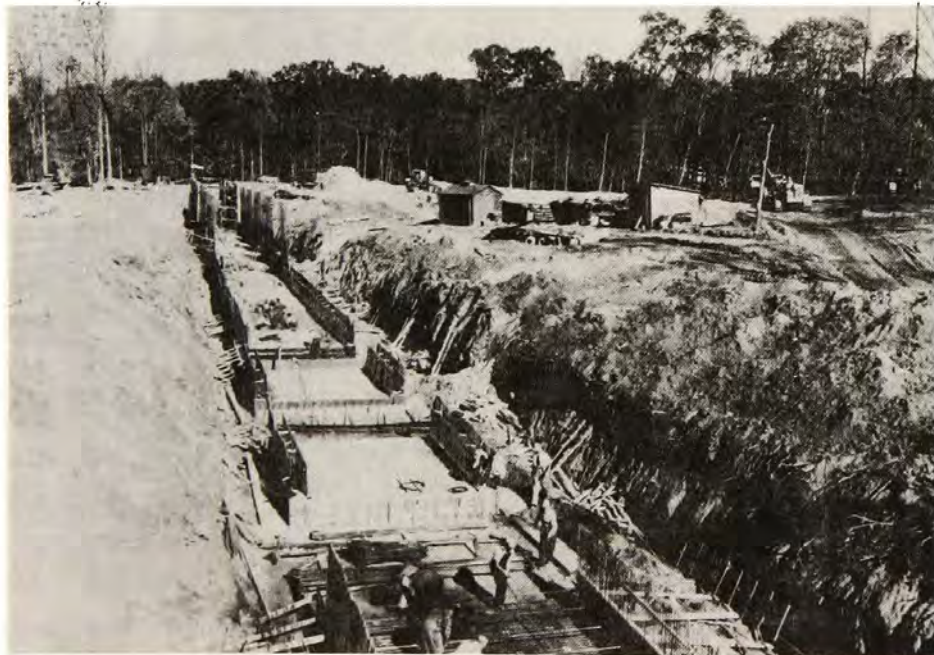
Figure 28. Sides of the 635-foot tank beginning to take shape. To the right, grading for shore processes test basin is underway, 5 November 1949.
