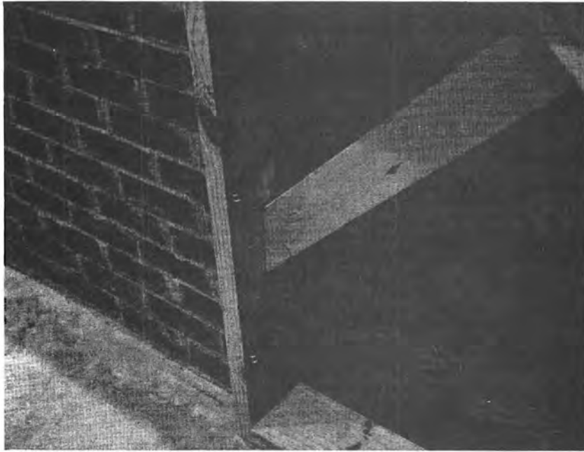
Figure 33. Springs used to pull the closure against the wall and down to the floor
